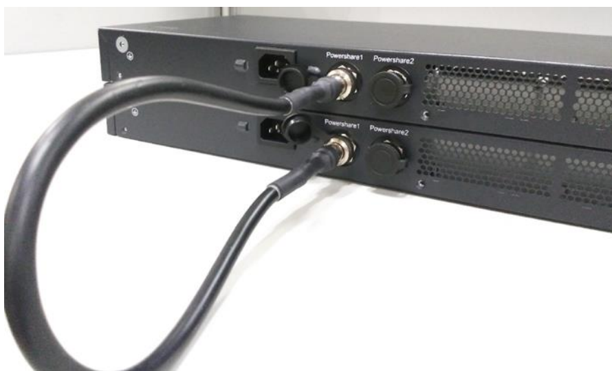
Figure 3-9 Connecting Cables between Two Switches
